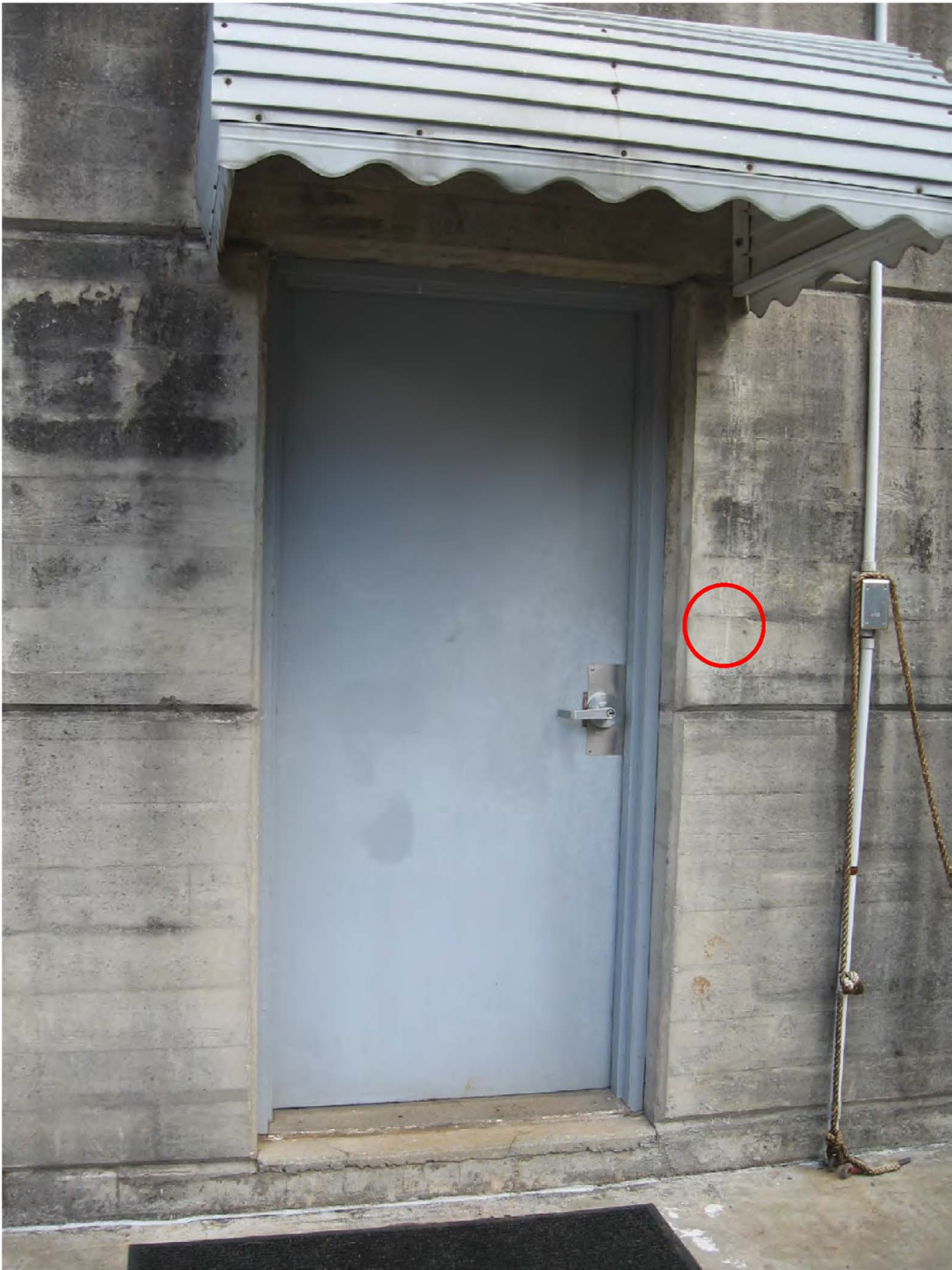
Figure 21: Exterior of existing entrance on the south elevation of the powerhouse which opens onto the switchyard. An entry card reader will be installed on the exterior wall beside the door (location circled in red).
