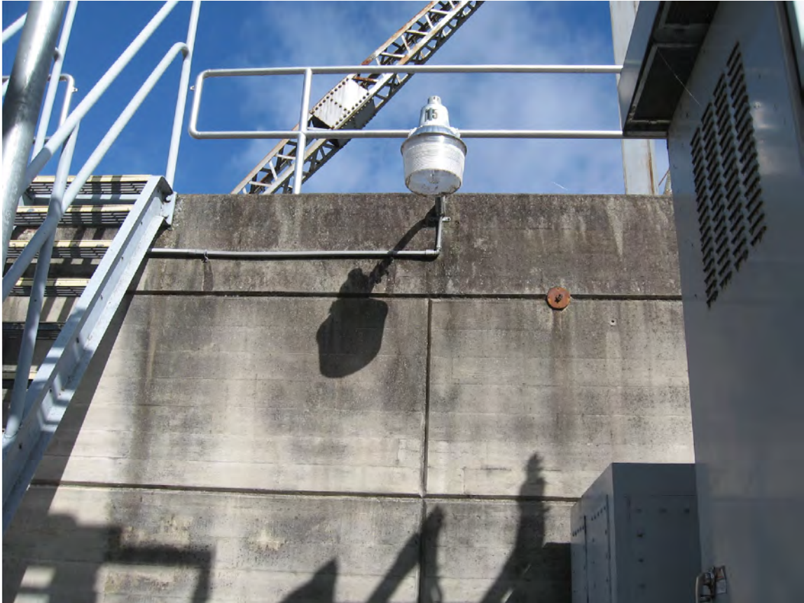
Figure 28: A new security camera will be added to the south elevation of the powerhouse at this location to monitor the transformer yard cable hatch and switchyard area.
