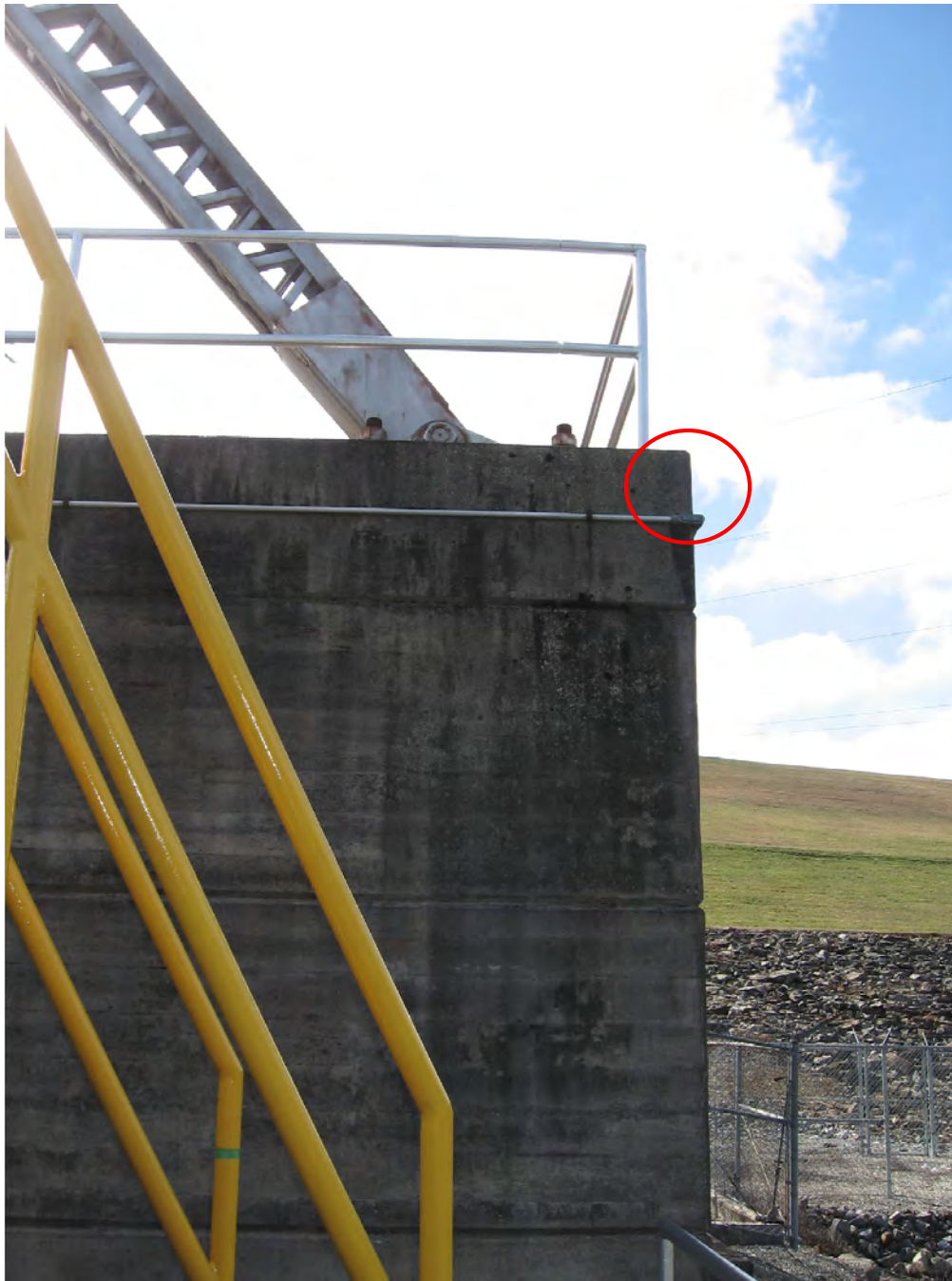
Figure 26: In order to monitor the west and north elevations of the powerhouse and the penstock ladder hatch location, a new security camera will be added at the northwest corner of the powerhouse. This location is shown as the red circle.
