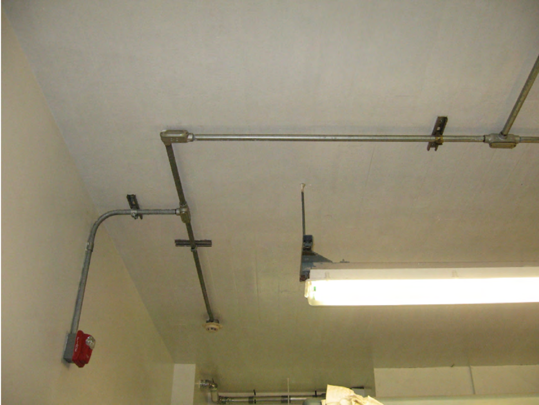
Figure 20: Proposed ceiling location of the security camera for the control room's west door. The wiring for the camera will follow the existing conduits as much as possible.
