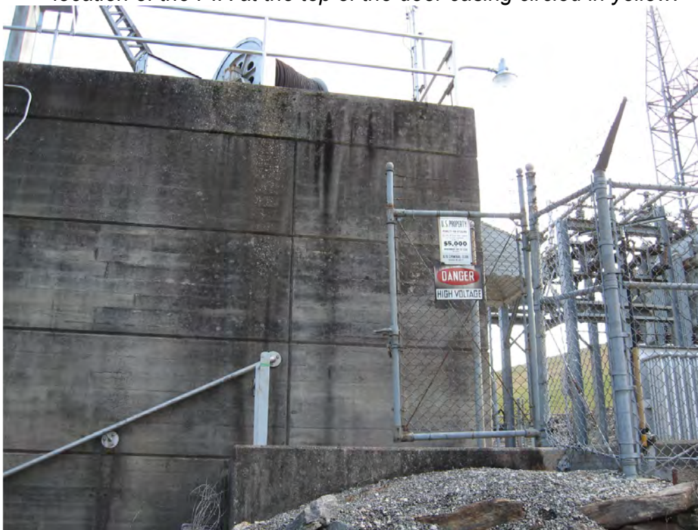
Figure 24: View of the penstock ladder hatch location on the west elevation of the powerhouse. A new chain link fence will be extended to enclose this area.
