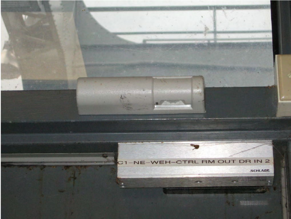
Figure 11: Close-up view of the passive infrared (PIR) sensor on the interior of the door. Similar sensors will be added to the interiors of the control room doors at the Chatuge Powerhouse.
