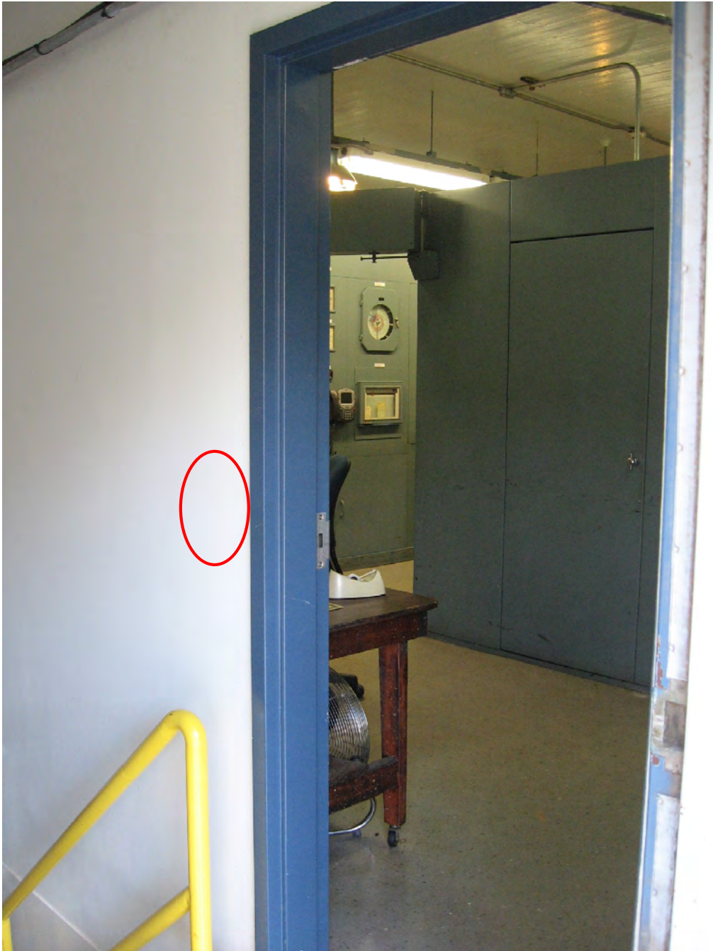
Figure 19: Interior of the powerhouse control room, viewing the location of the entry card reader to be installed (red circle).
