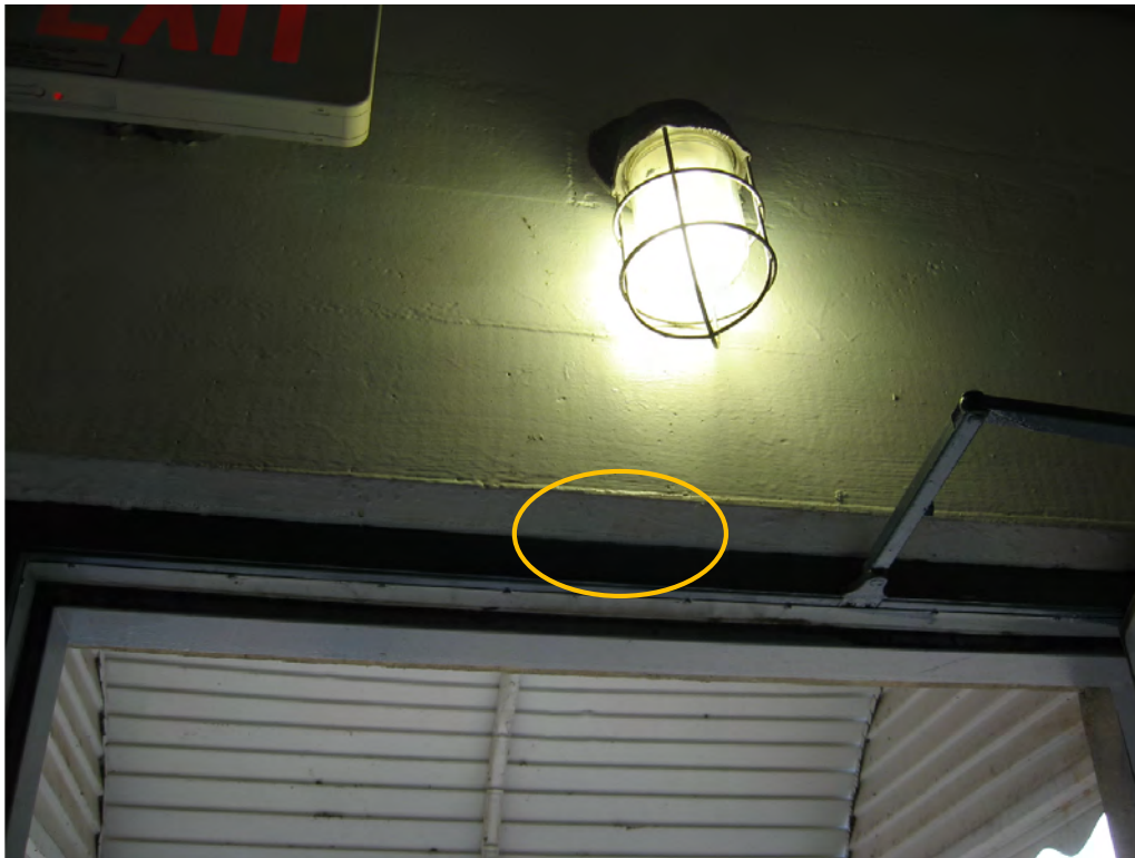
Figure 23: This view shows the interior of the south powerhouse door with the location of the PIR at the top of the door casing circled in yellow.
