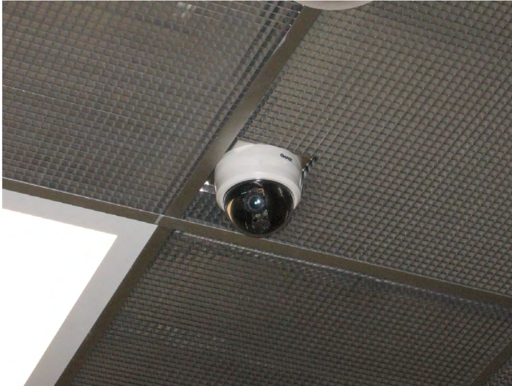
Figure 13: The new security cameras to be installed in the powerhouse will be similar to this one in use at the Wheeler Powerhouse in Alabama. This is a ceiling-mounted example.
