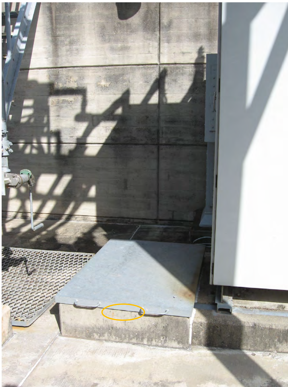
Figure 27: The transformer yard cable hatch will be retrofitted with a new alarm contact and this location is shown as the yellow circle.
