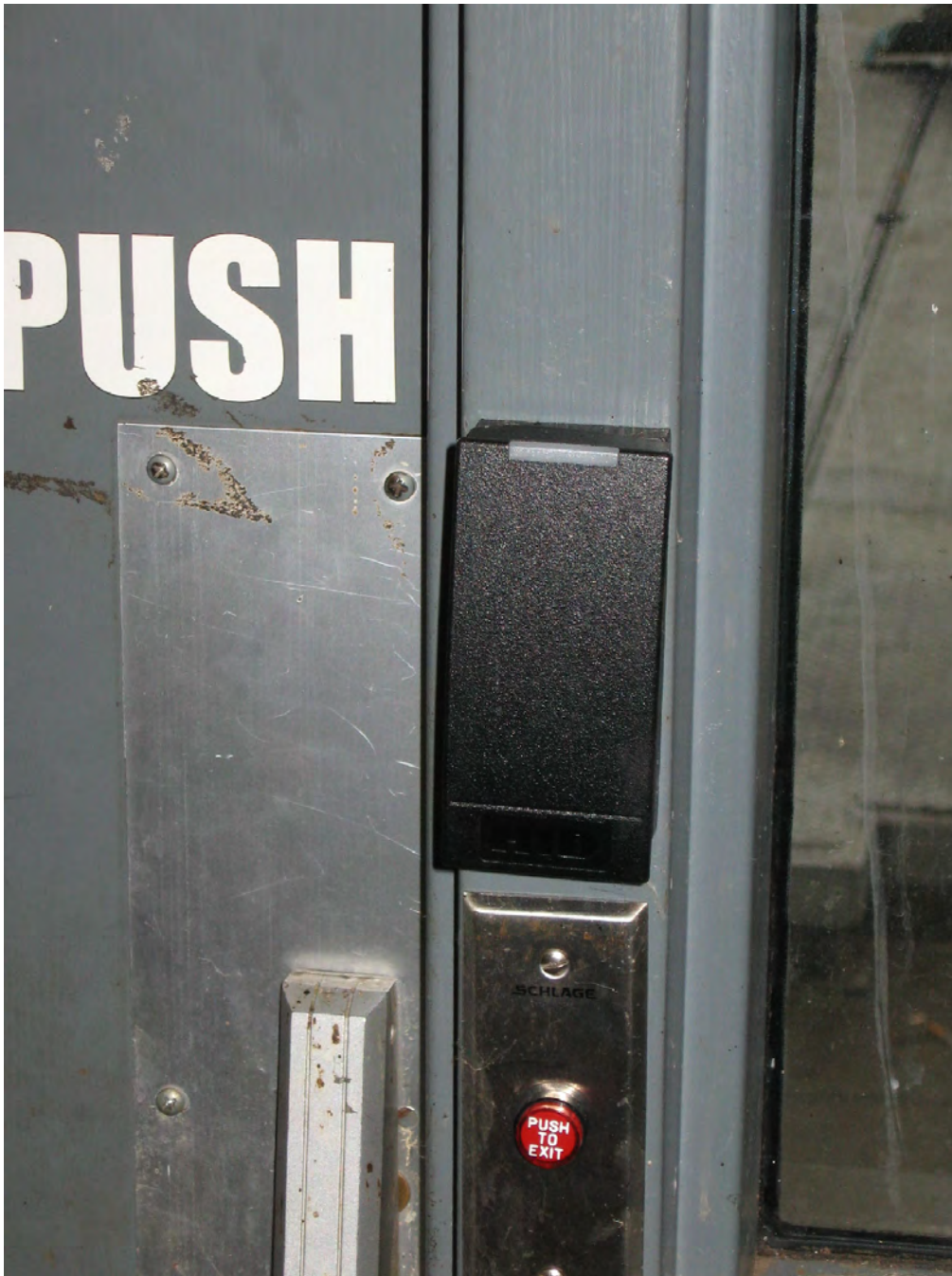
Figure 9: A close-up view of the card reader similar to those to be added at the Chatuge Powerhouse.
