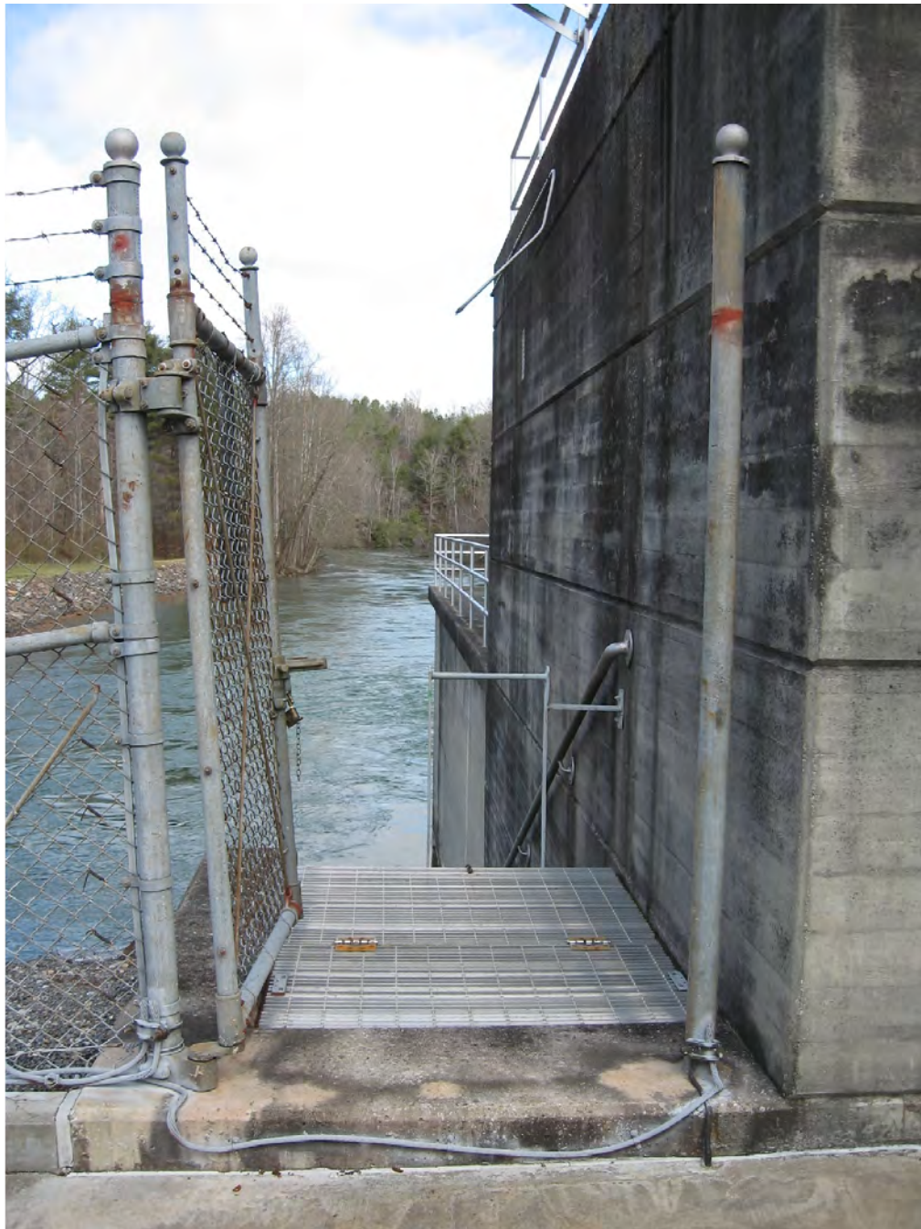
Figure 25: View of the penstock ladder hatch location on the west elevation of the powerhouse. A new chain link fence will be extended to enclose this area. The new fence will be beyond the metal hatch shown and will abut, but not be connected to, the exterior wall of the powerhouse.
