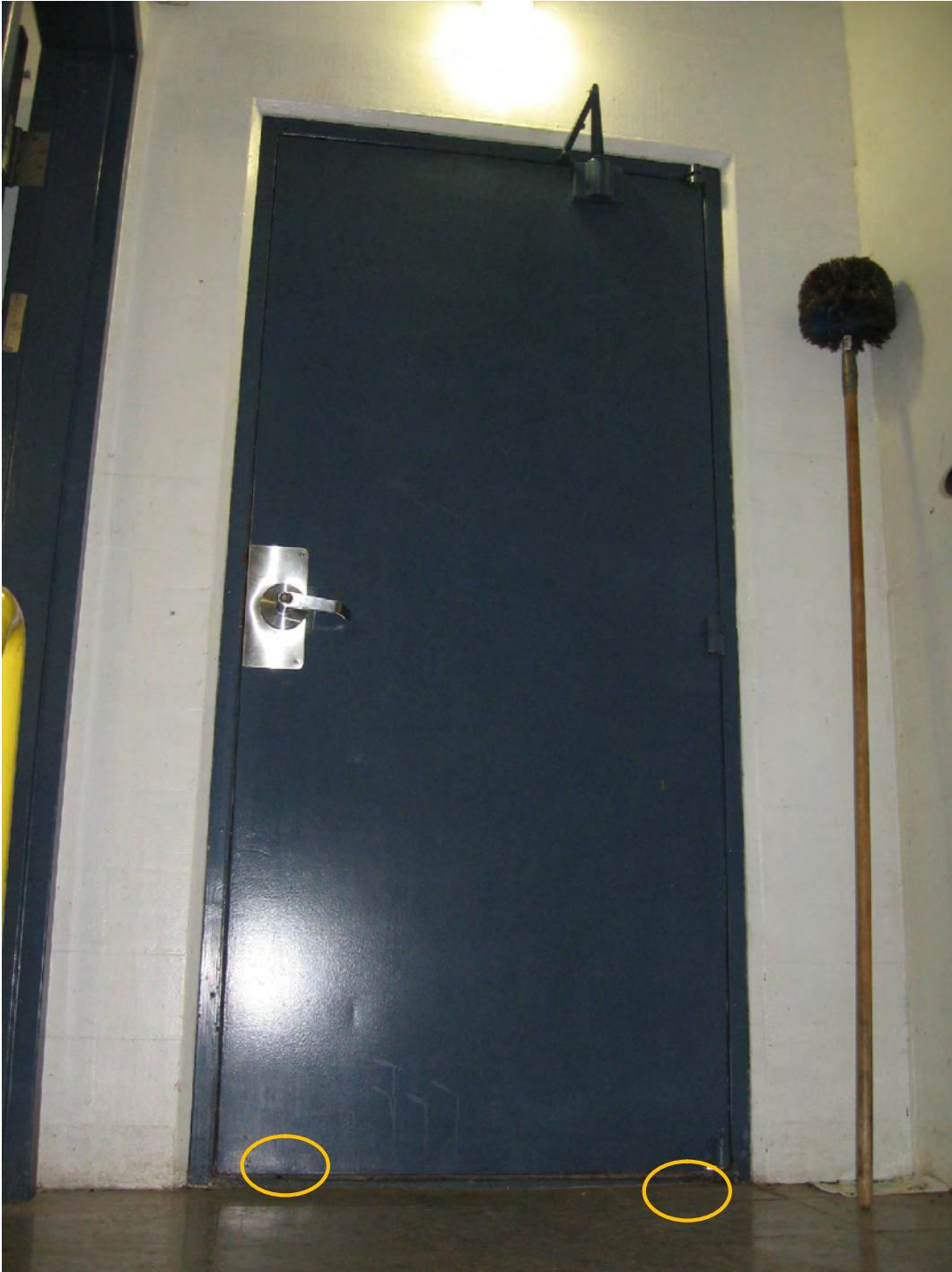
Figure 22: This view shows the interior of the door with the location of the floor-mounted alarm contacts circled in yellow.
