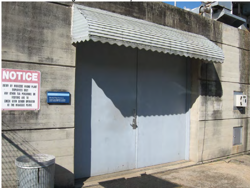
Figure 14: The main entrance to the control room on the east elevation of the powerhouse has steel double doors.
