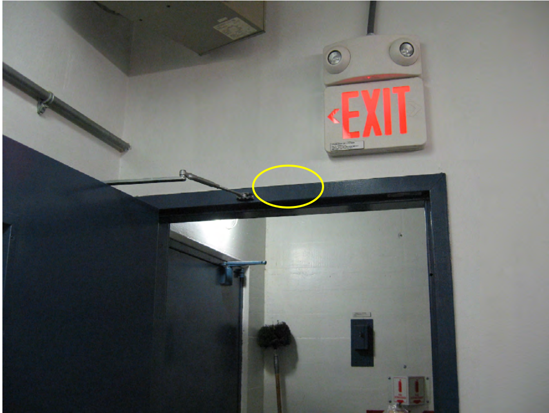
Figure 18: Interior of the powerhouse control room, showing the location of the PIR sensor to be installed above the control room's west interior door (yellow circle).
