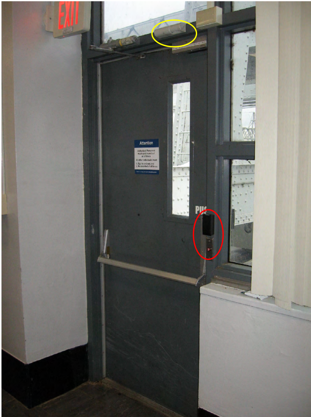
Figure 8: The new passive infrared (PIR) sensors and entry readers to be installed in the powerhouse will be similar to these at the Wheeler Powerhouse in Alabama. The red circle shows the reader with a push button shunt and the yellow circle shows the PIR sensor.
