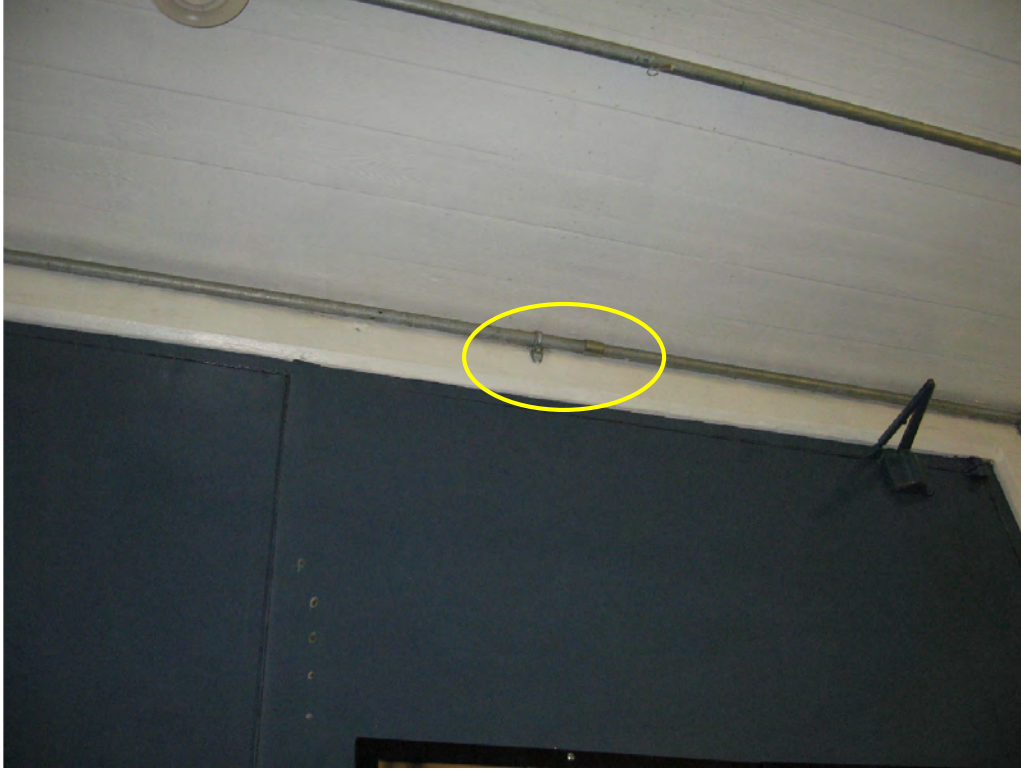
Figure 16: Interior of the powerhouse's control room with the yellow circle showing the location of the proposed passive infrared (PIR) sensor.
